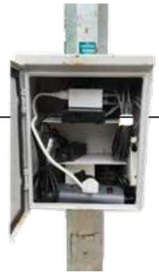
Outdoor CCTV Pole
